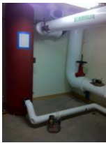
Plumbing components water hammer arrestors surge tanks under sink filters
