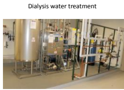
Dialysis water treatment
