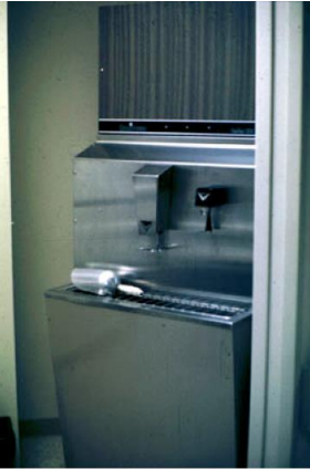
Ice machine maintenance •charcoal filters? •moldy storage bins
